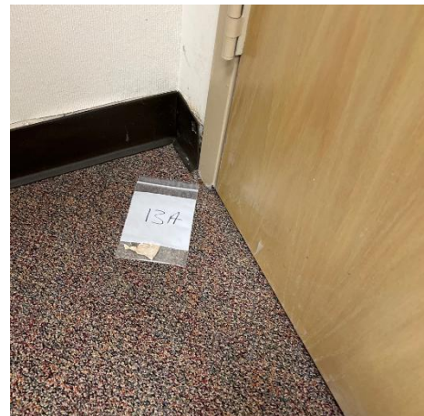
13A, Cove Base Adhesive, Meeting Room Connected to Printing Area
