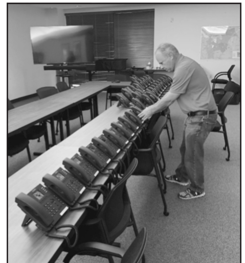
New phones during preparations for installation at the NEGRC by Business Telephone Systems of Athens.
